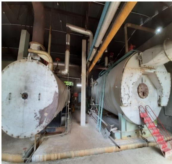
Figure 10: No railing for the service platform of boilers
