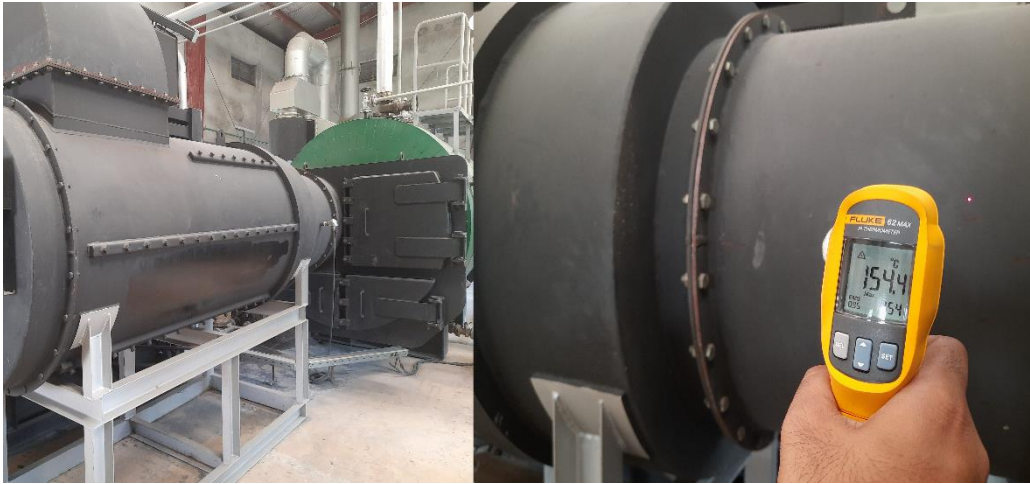
Figure 12: Uninsulated hot surface in the boiler room
