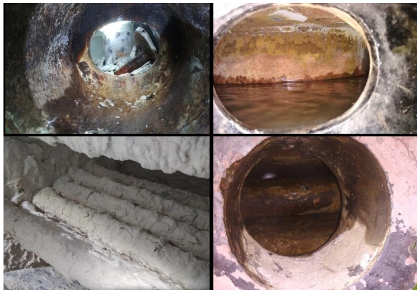
Figure 1: Corrosion of the metal and scale formation inside the boiler for using untreated water (Accord, 2019; Siraj et al. , 2023)
