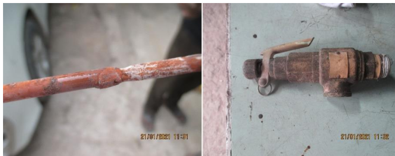
Figure 4: Lengthening the level sensor by welding (left), rusted stuck safety valve (right); observed during the Incident inspection by the RSC at Sincere Composite Ltd.
