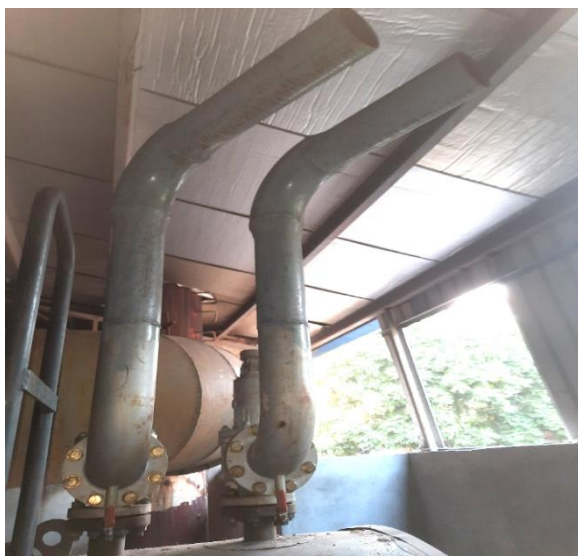
Figure 8: Safety valve discharge point inside the room
