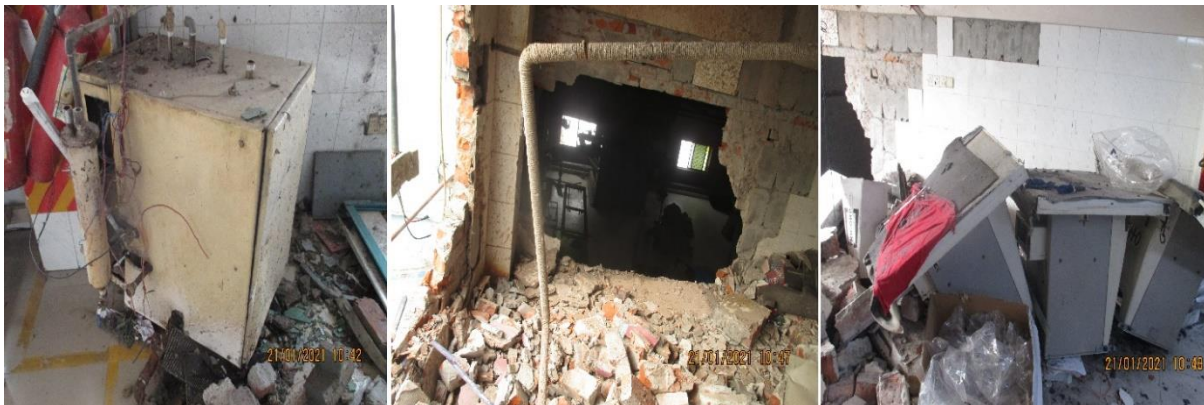
Figure 3: Mini-boiler (left), collapsed boiler room (middle), impact on the adjacent production floor (right); observed during the Incident inspection by the RSC at Sincere Composite Ltd.
