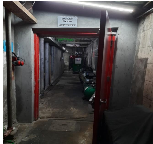
Figure 11: Inadequate clearance, obstructed ventilation
